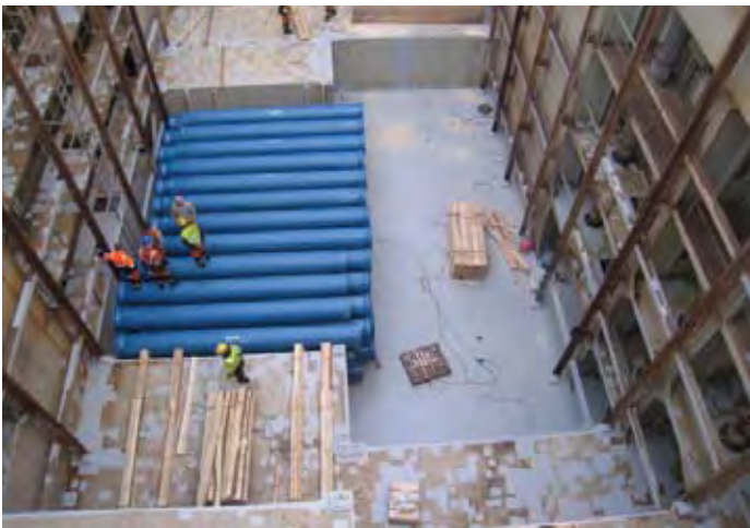
^ Pipes stowed correctly
