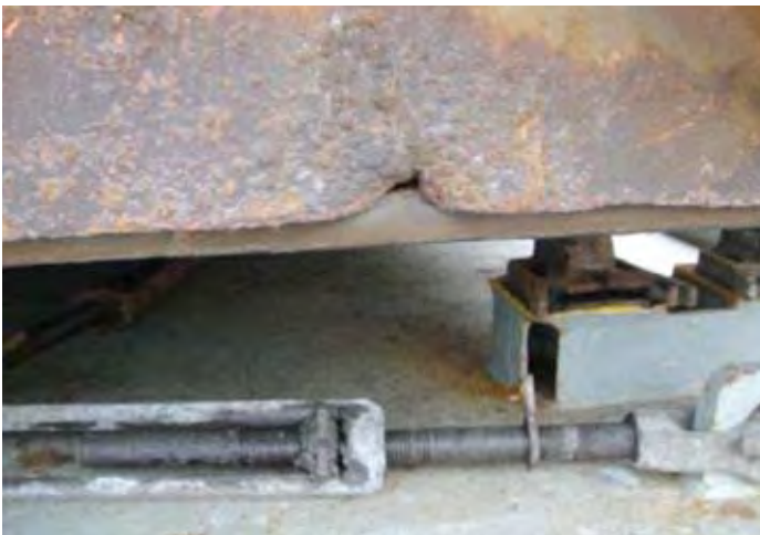
^ Damaged hatch cover edges would allow water ingress – sufficient to cause water damage to water-sensitive cargo
