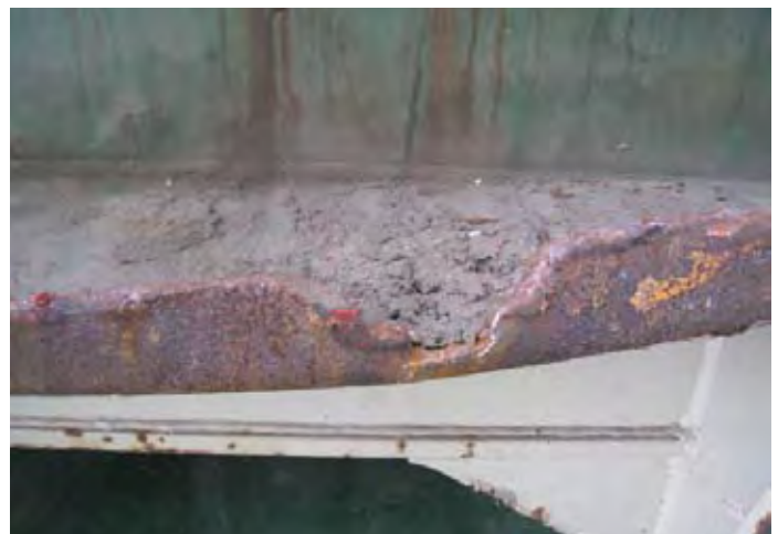
^ Damaged channel bars – potentially allowing water ingress
