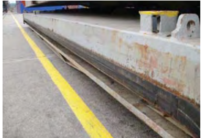
^ Hatch cover longitudinal joints such as these would have to be in good condition to prevent water ingress
