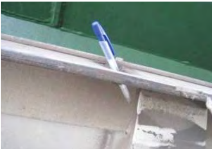
^ A damaged seal, which will allow water ingress
