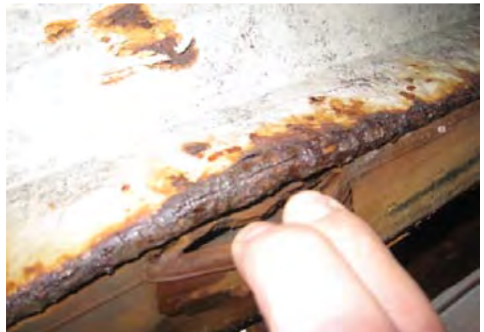
^ Damaged packing rubber seals
