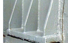
Damaged resting pad.
