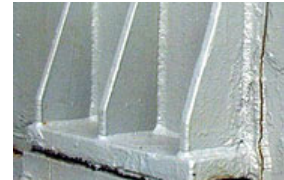
Damaged resting pad.
