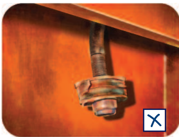
Cleat – damaged washer
